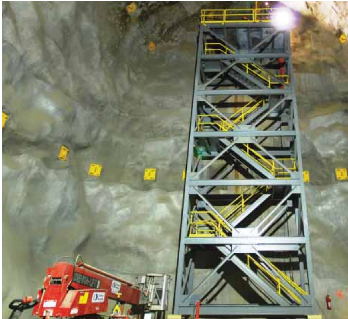
Phase one's main hall is rectangular in shape with barrelled walls and roof for structural support.
